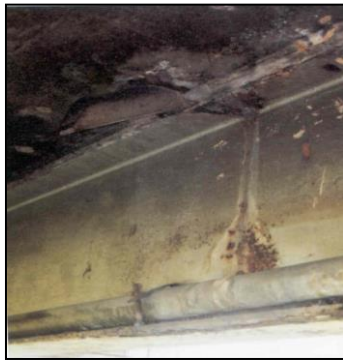
Gambar 4-6 Bocornya pipa drainase
