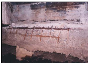
Gambar 4-10 Korosi tulangan abutment.
